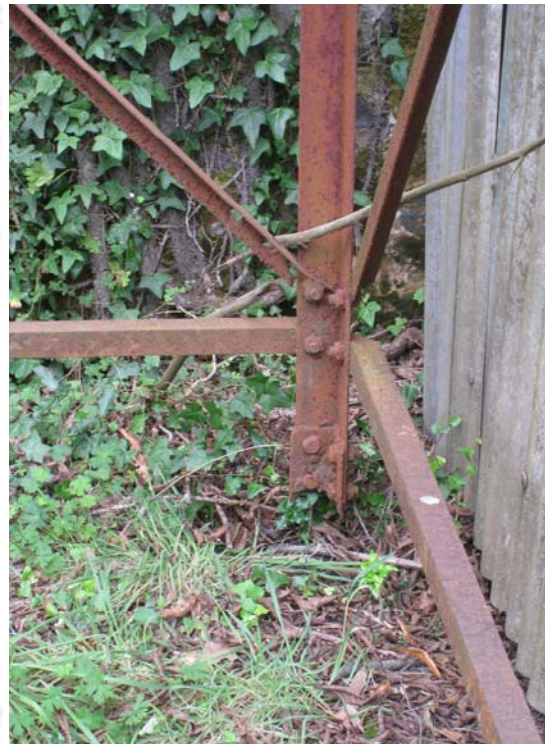
Figure 22: Leg at base of tank stand rusted off at ground level.
