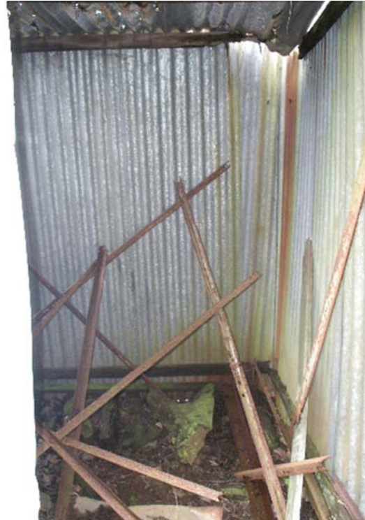
Figure 16: Corroded framing members. (Source: Hughes Trueman 2009)
