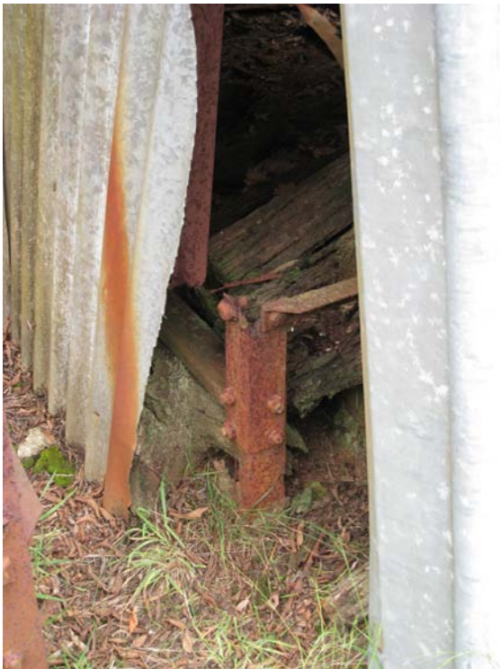
Figure 21: Severed leg at base of tank stand.
