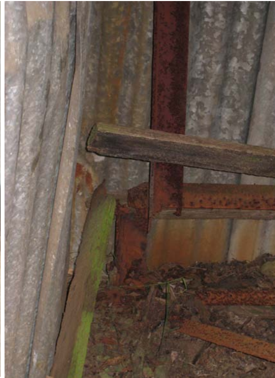
Figure 20: Severed leg at base of tank stand.
