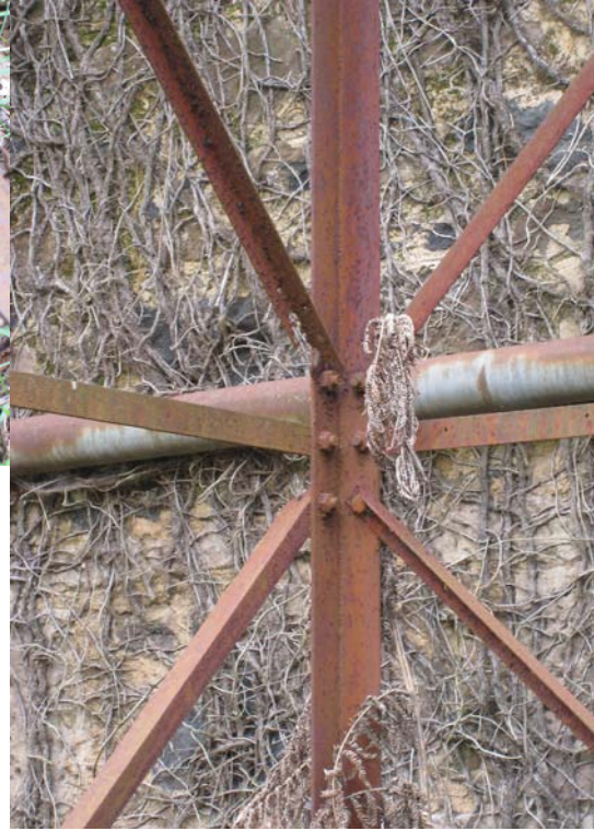
Figure 24: Detail of the framing. Note the corrosion in the diagonal bracing.
