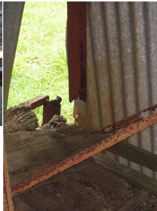
Figure 18: Severed leg at base of tank stand (of the eight tank stand legs, only three are providing support).
